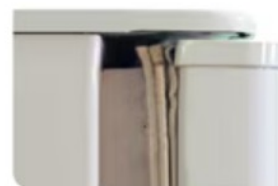
Mould, which spreads on the door seal, will cause distortion
